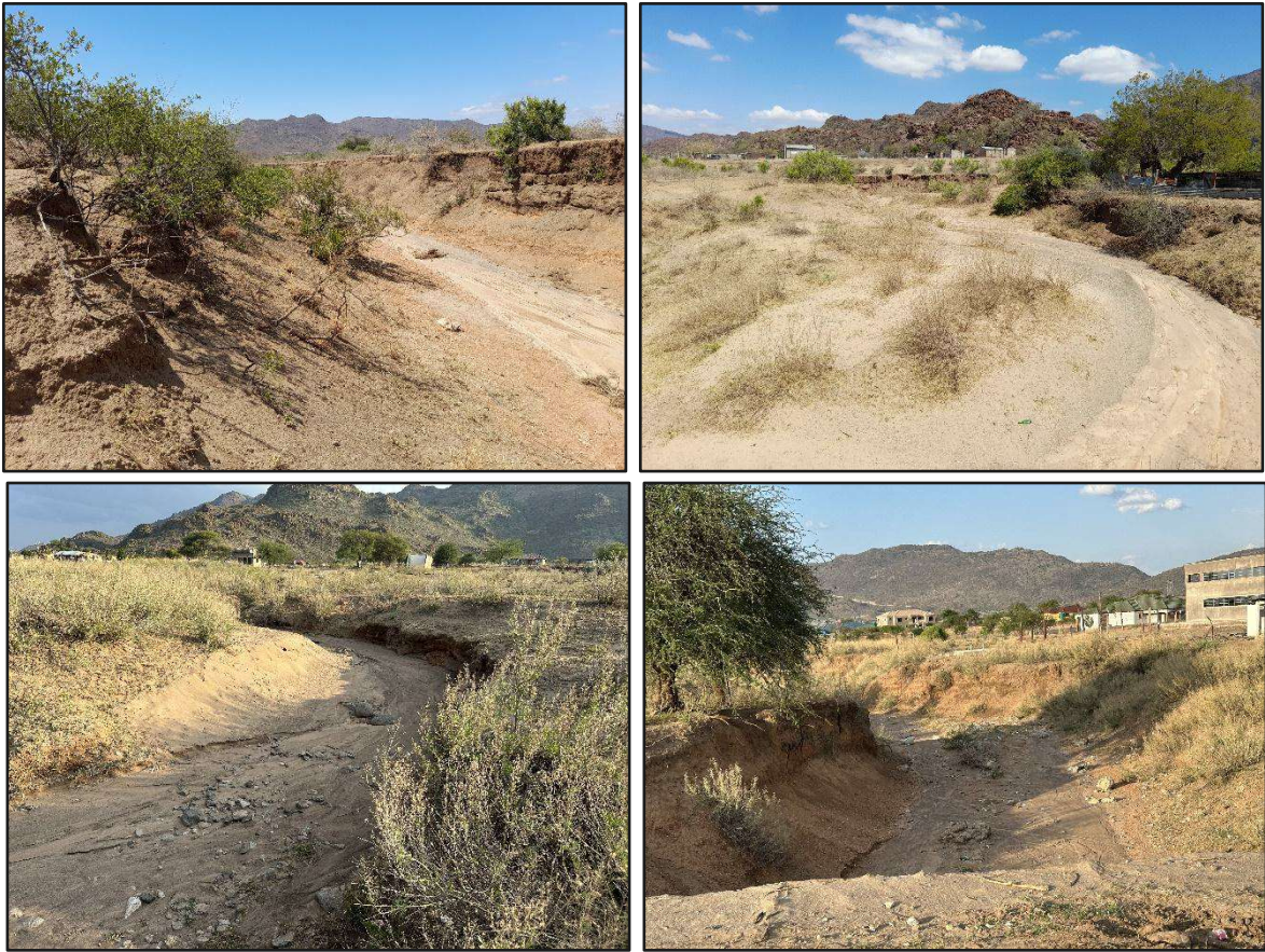
Photograph notes: Top left: Channel bed and banks of the drainage line near access point 1-17, showing excessive bank erosion; Top right: The same drainage line upstream of the road and access point illustrating very limited residual vegetation cover in the riparian zone; Bottom left: The drainage line at access point 2-08 with the only remnant vegetation being herbaceous shrub species which are not browsed by livestock ; Bottom right: The reach of the drainage line downstream of the road at access point 2-06 showing limited woody vegetation and housing in the immediate catchment of the reach.
