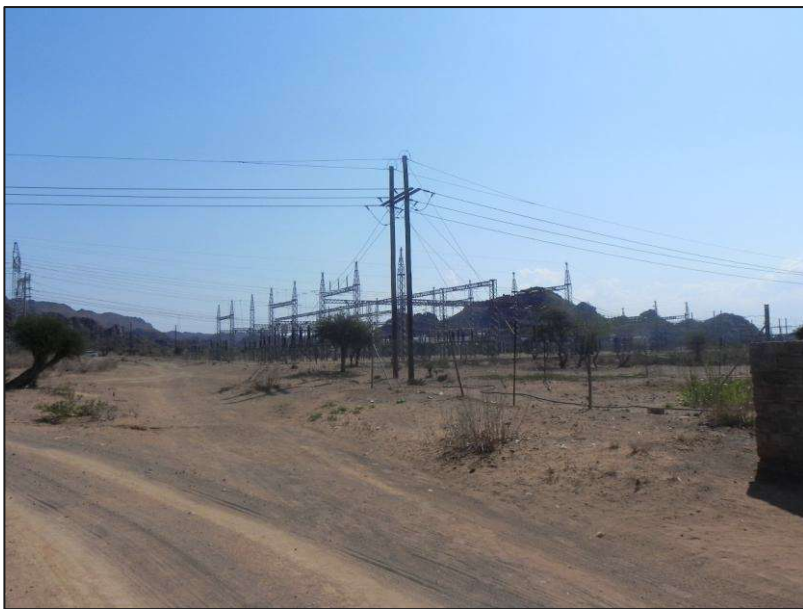
Figure 7-89: Eskom Middelpunt substation located close to the settlement of Zeekoegat.
