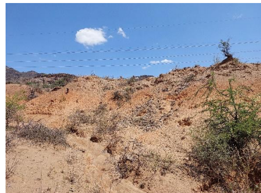
Figure 9: Example of the Erosion Gulleys present in the Project Area
