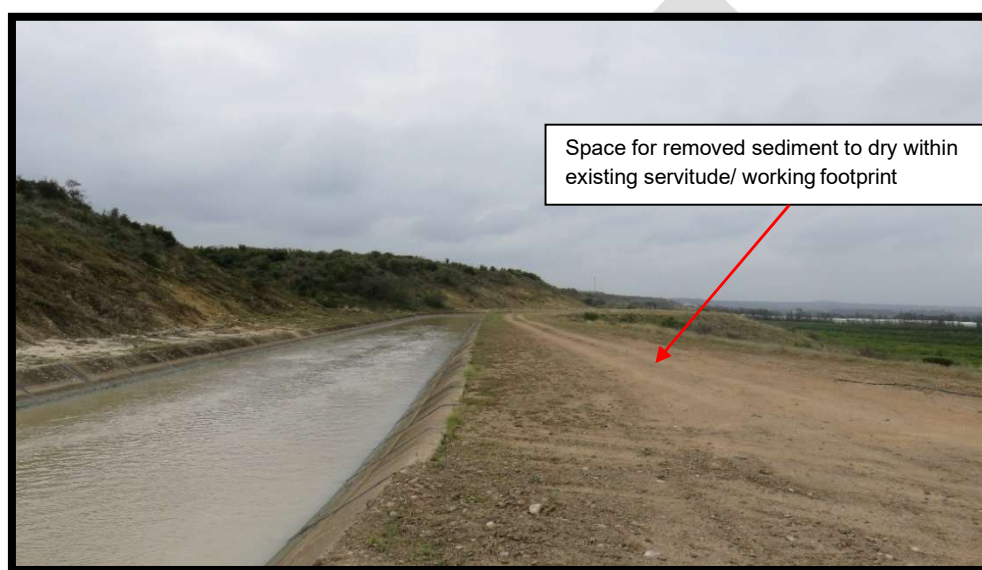
Figure 24. Example of existing LSRWUA canal servitude (photo: T Duvenhage)
