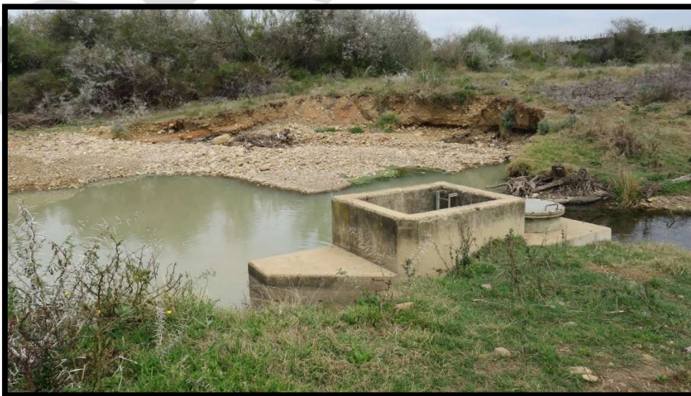
Figure 22. Typical scour structure at the Enon syphons (photo: T Govender)
