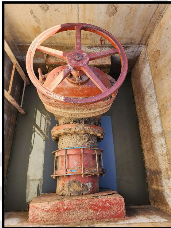
Figure 23. LSRWUA Valve chamber (photo: C Jonker)
