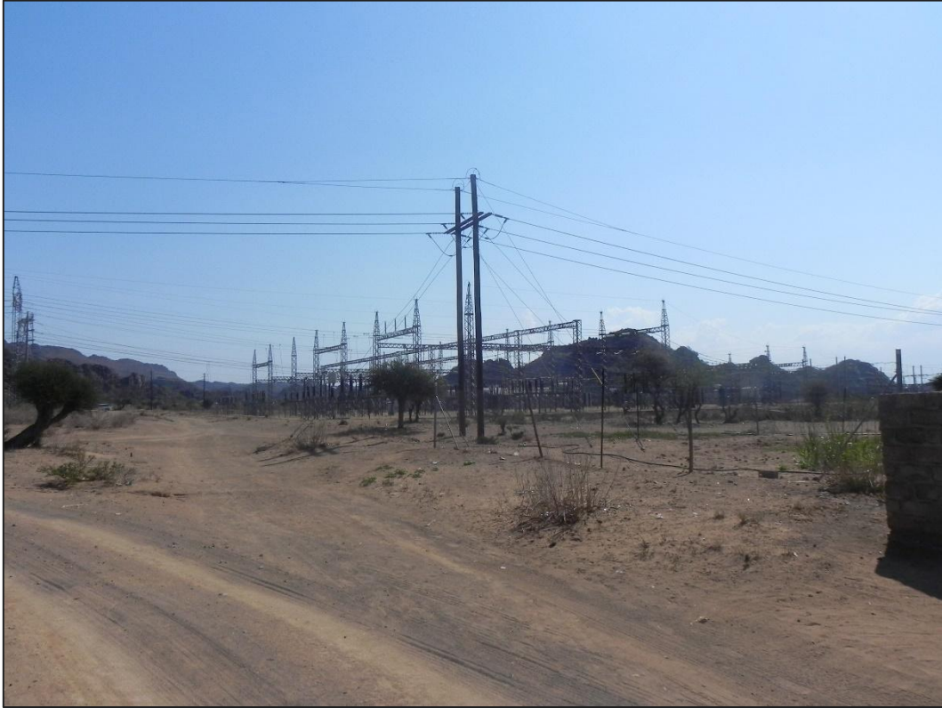
Figure 19: Eskom Middelpunt substation located close to the settlement of Zeekoegat
