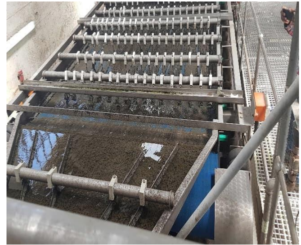
Belt Presses - Dewatering
