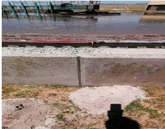
Secondary Settling Tank
