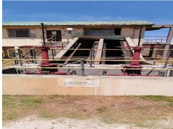
Screw Lift Pump Station
