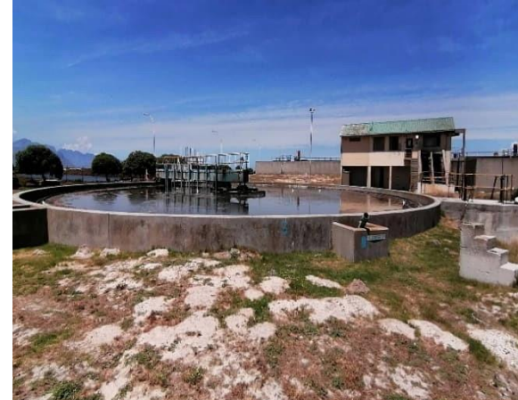
Secondary Settling Tank
