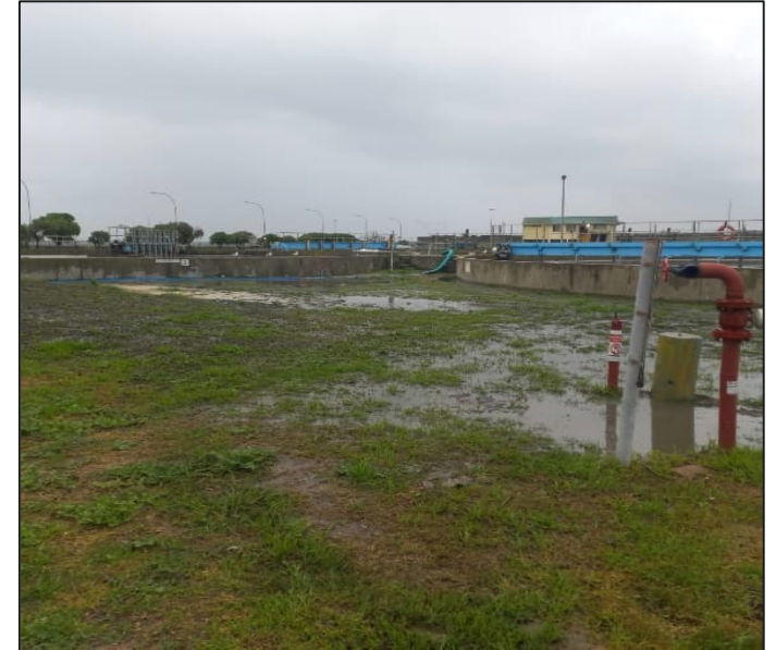
Spillages at SST's area
