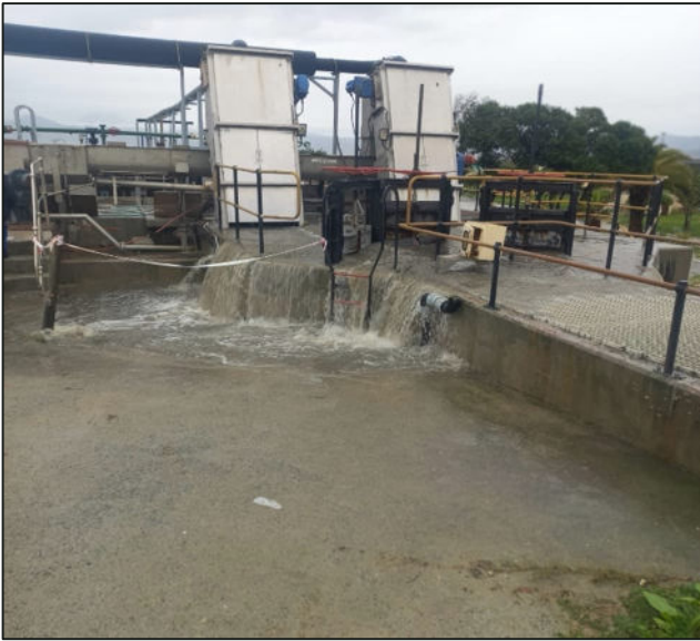
Inlet works flooding
