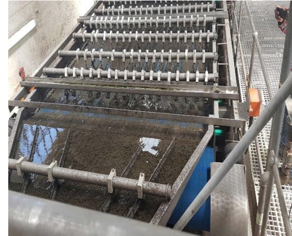
Belt Presses - Dewatering
