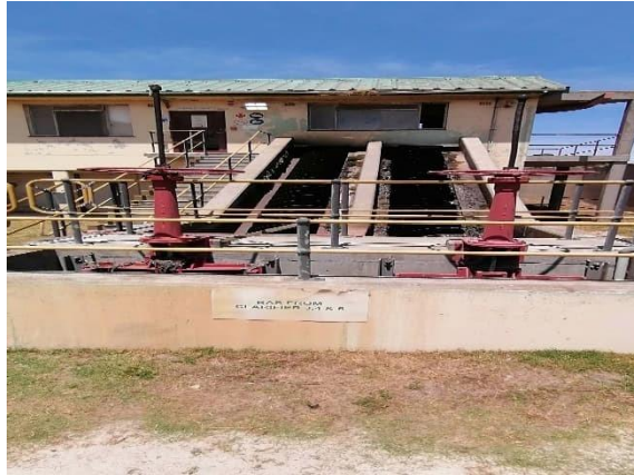
Screw Lift Pump Station
