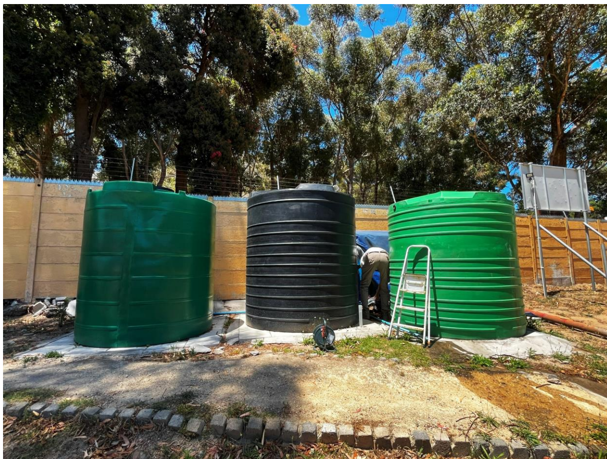
Photo 10: Storage tanks prior for borehole HBH1
