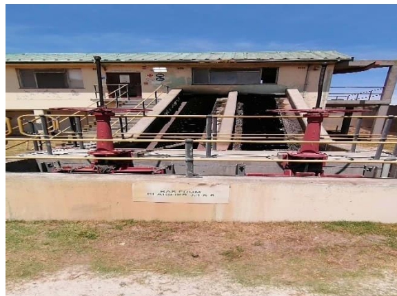
Screw Lift Pump Station
