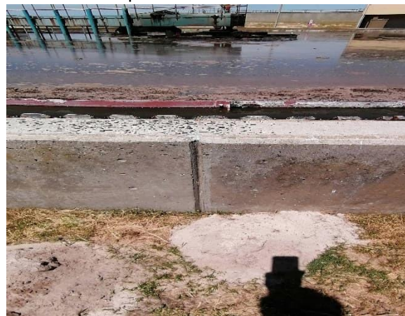
Secondary Settling Tank
