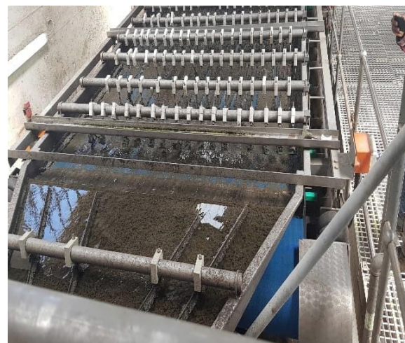
Belt Presses - Dewatering
