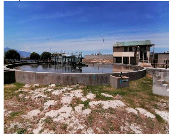
Secondary Settling Tank
