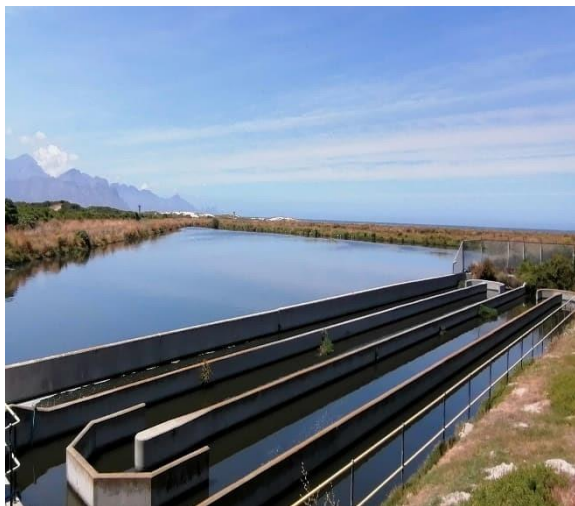
Chlorine Contact Tank
