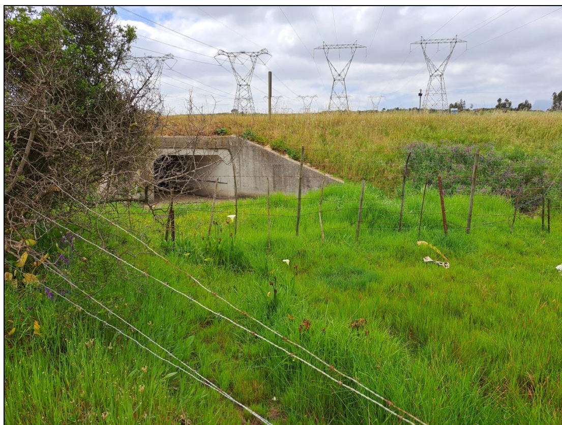
Figure A4.8.8 Culvert under the R304, carrying the watercourse (Aquatic Ecosystem 3) under the road.
