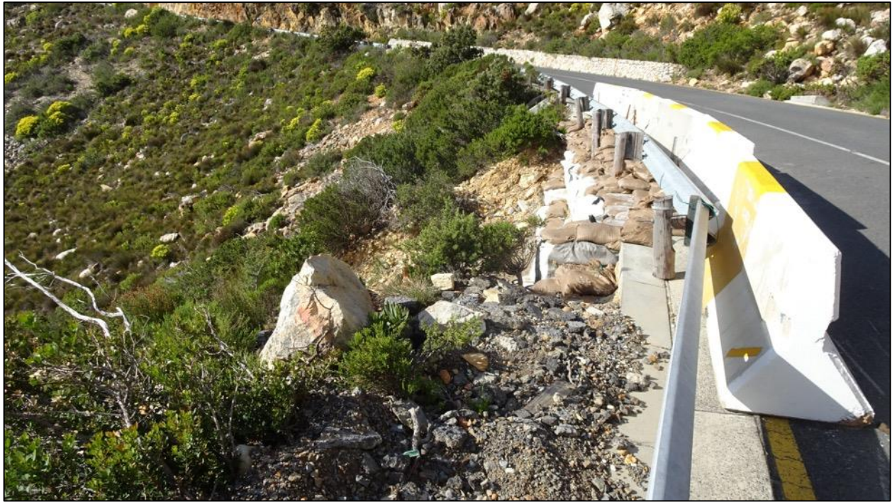
Figure 17. The upper limit of the erosion zone along the road edge.
