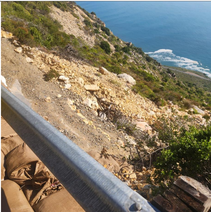
View of the Kogelberg Sandstone Fynbos and the damage to the slope 1 area
