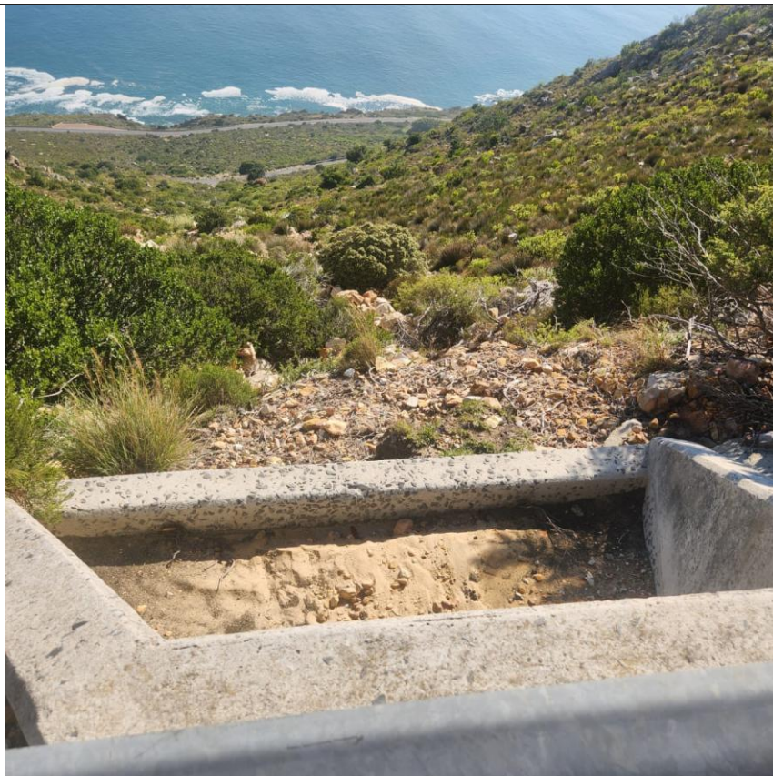
Example of the blocked culvert and Kogelberg Sandstone Fynbos on the proposed slope 1 rehabilitation area
